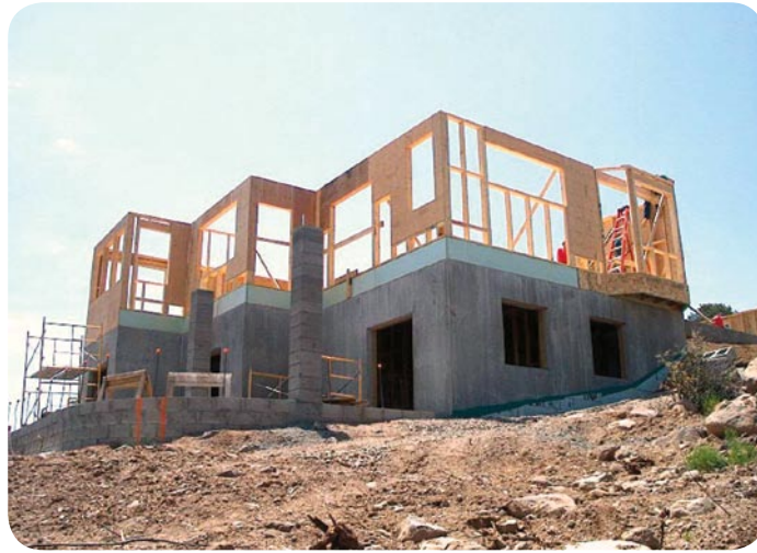
Energy efficient features in the Longview House include insulated, prefabricated concrete walls; advanced framing, and rim joist insulated with rigid insulation.
