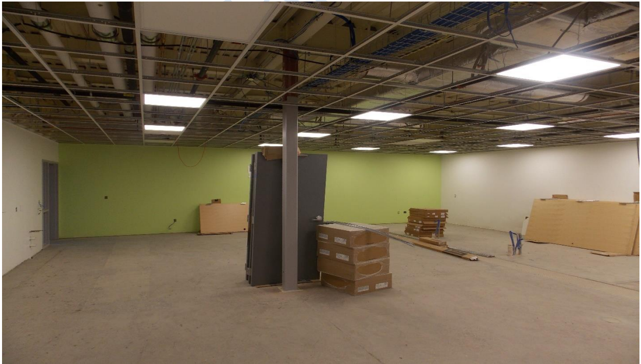
Ceiling Grid and Lighting in Biology Lab
