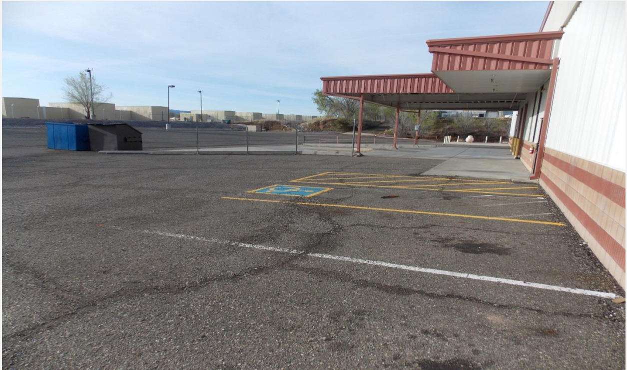
CTEC Parking Lot Deterioration
