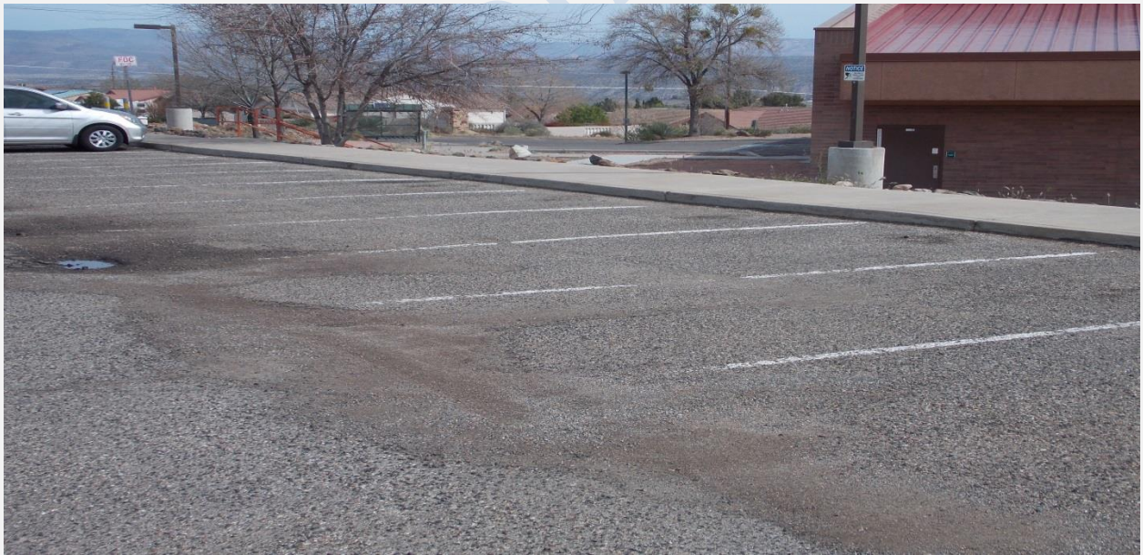
Verde Valley Campus Parking Lot Deterioration
