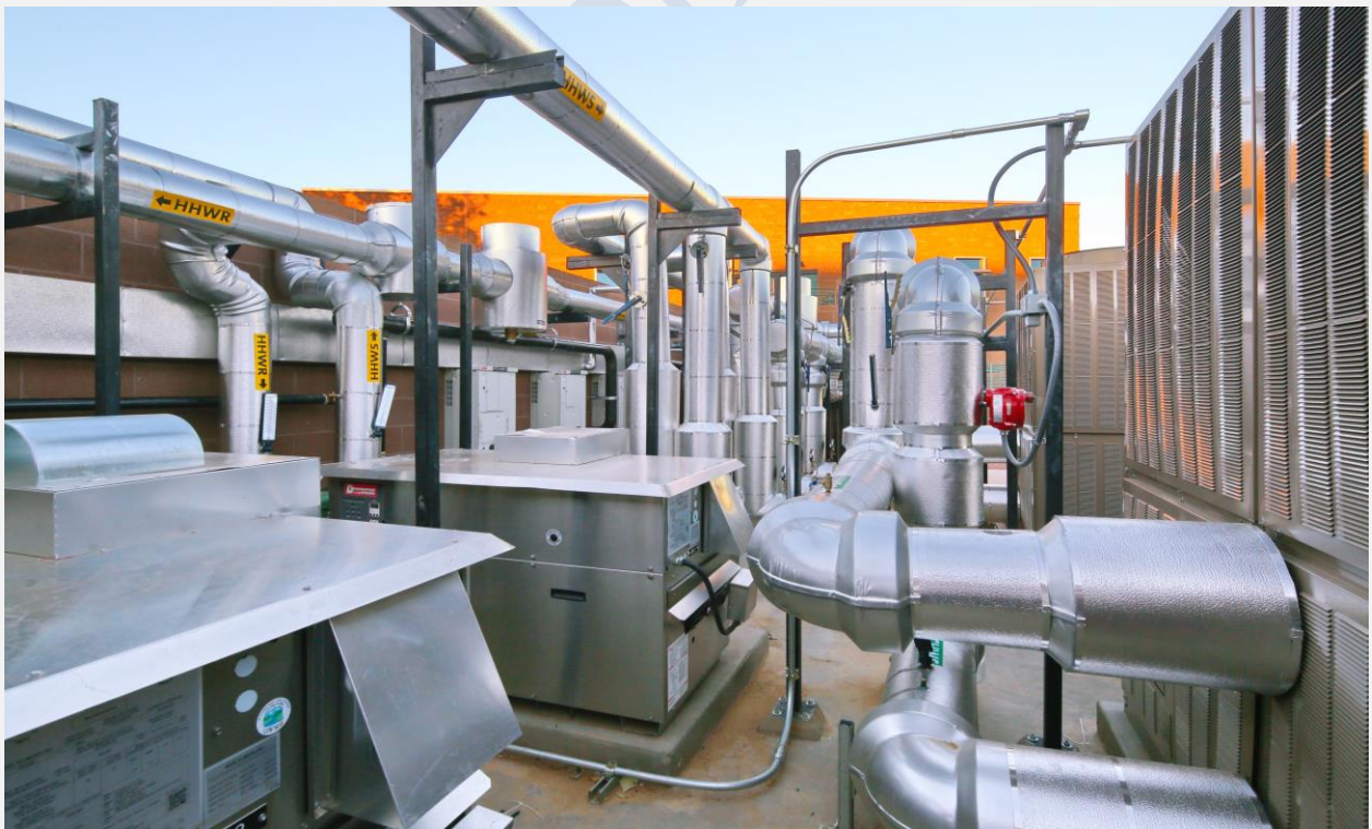
New Central Plant
