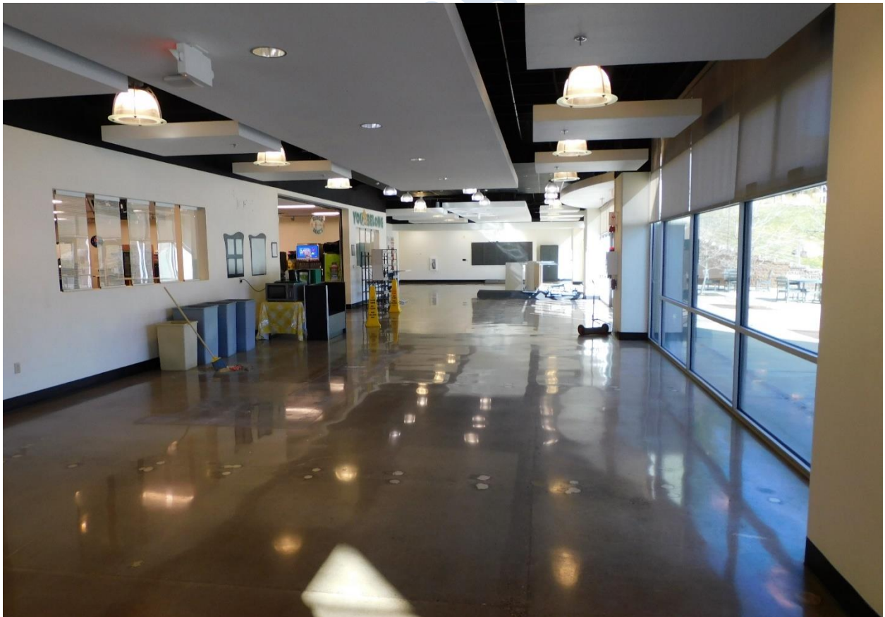
Floors prepped for new furniture to arrive the first week of January
