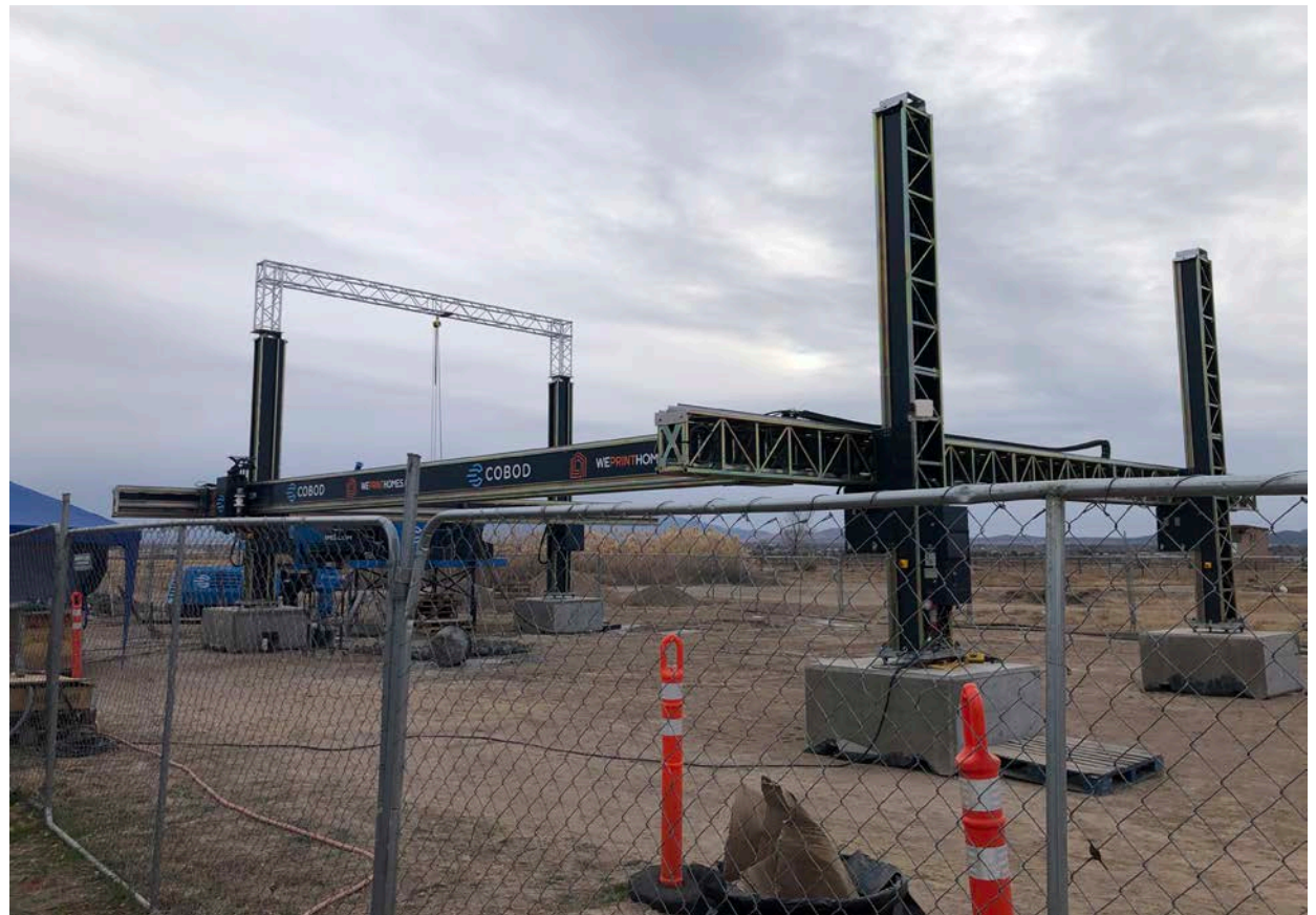
The construction lab is building a 3D printing house on site at Chino Valley center
